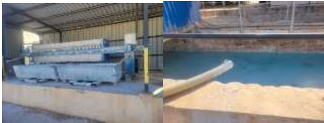
Figure III-2: The lime milk waste processing area
