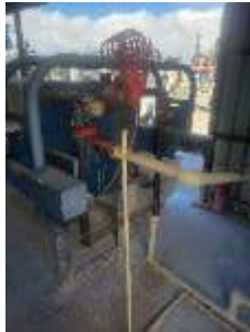
Figure III-5 : The filtration system
