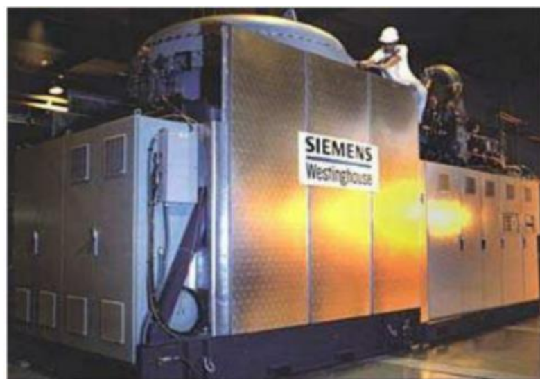
Figure III-14: L'installation Siemens-Westinghouse de Irvine (220 kW) (2002). [53]
